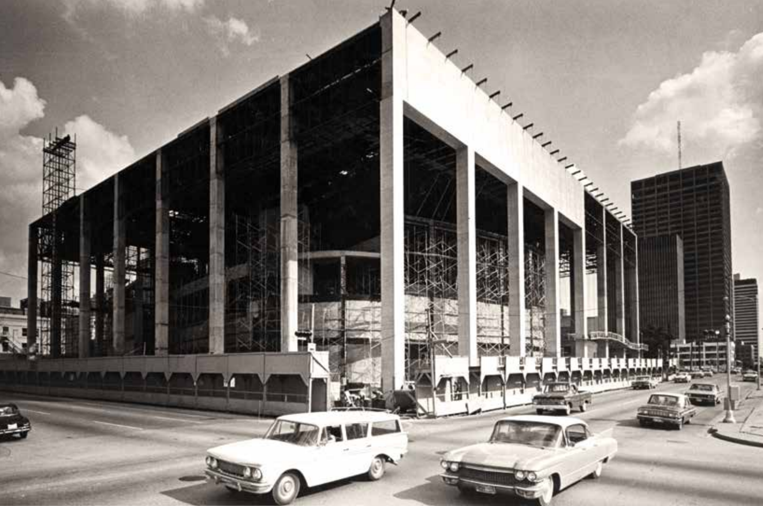
In 1966, 40 workmen spent ten months attaching the marble to Jones Hall's exterior and interior walls. The city block's nine-foot change in elevation required each of the columns around the building's perimeter to be a different length.
